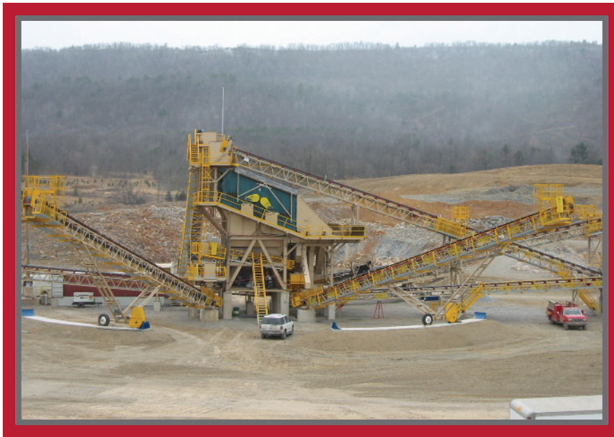
Hawbaker uses a mobile crusher and conveyors, instead of conventional haul trucks, and a wireless control system from Rockwell Automation that eliminates the need for a permanent control room or a dedicated operator.
