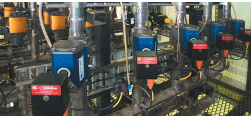
Over 500 valves (pictured) control and regulate oil flow about the Goodman Fielder Footscray site, via a maze of piping spools and tanks.
