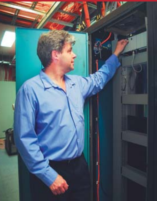
Goodman Fielder state operations manager, Greg Langusch, inspects one of the site's many Allen-Bradley PLC controllers.
