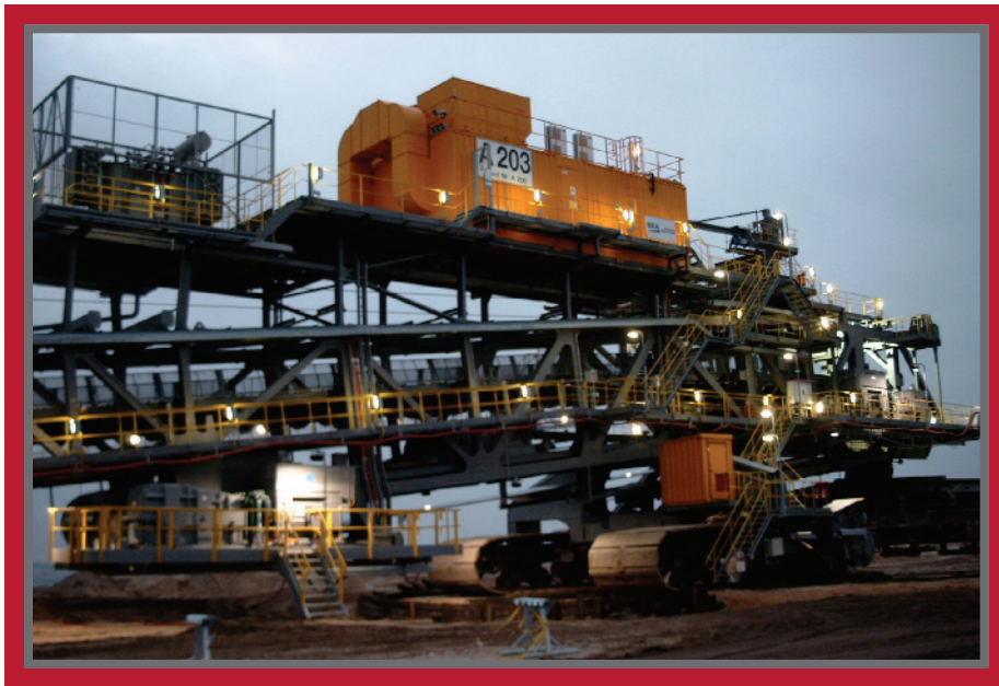
The mobile conveyor head station with limited footprint and acceptable weight for the complete drive system of up to four 2MW variable speed drives including transformer and switchgear.
