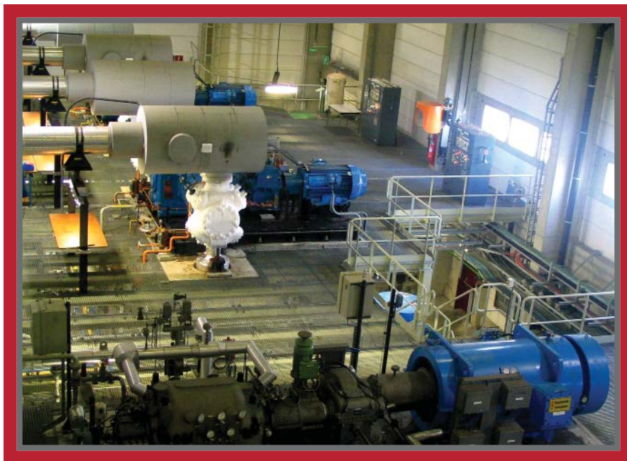
A medium voltage drive was installed on two of the five pumps and on the compressor providing the return gas to the ships' tanks. The compressor and the ice on the unit can be seen in the centre of the photograph.
